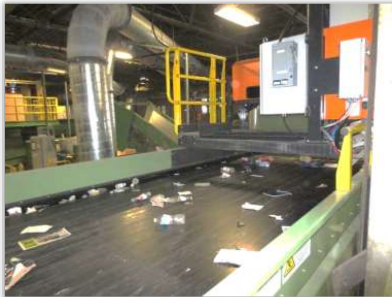
Figure 3: New Optical Sort Equipment
