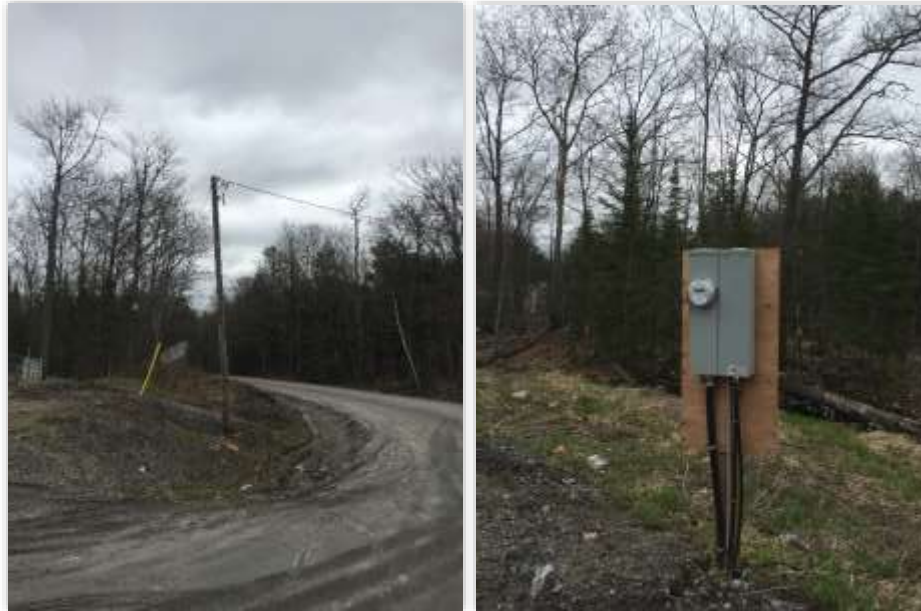
Figure 2: Photograph of hydro grid connection and metre
