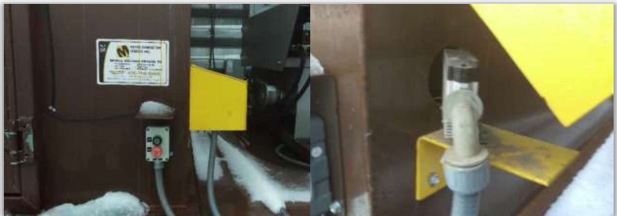
Figure 3: Optical Beam Sensor Installation
