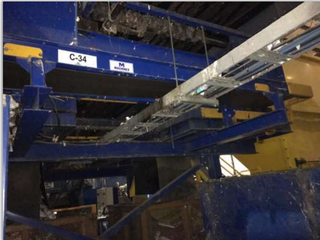
Figure 5: Container Return Conveyor
