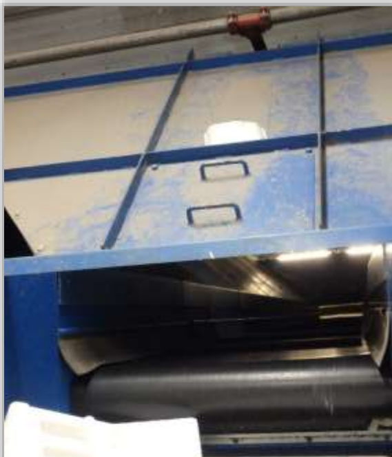
Figure 3 Infeed Conveyor from Container Sorting Station
