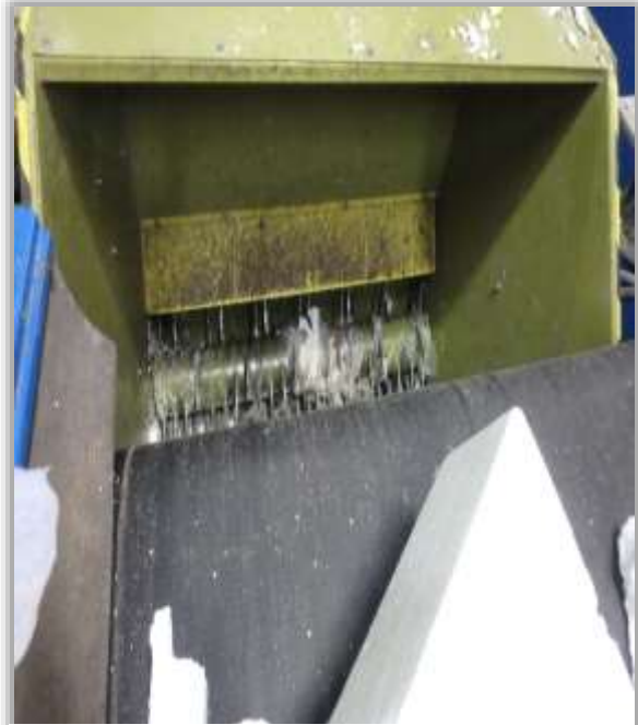
Figure 4 Infeed Conveyor to PDS Crusher
