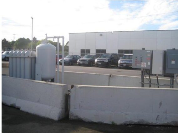
Figure 4: Ellesmere Yard CNG Fuelling Station
