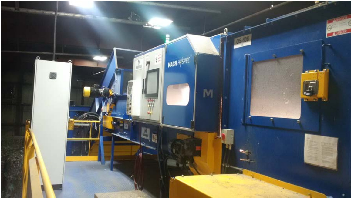
Photo 2 - Depicts the main optical processing unit that was installed
