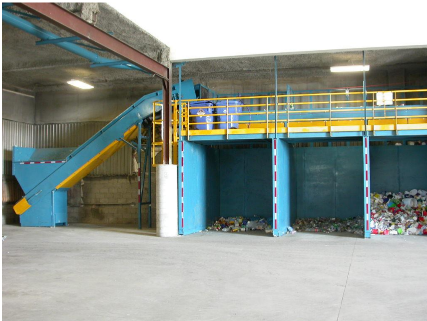
Photo of the right hand side of the new container line that was installed at the Recycling Center at 112 Patton Street, North Bay, Ontario. It indicates the inclined conveyer belt.
