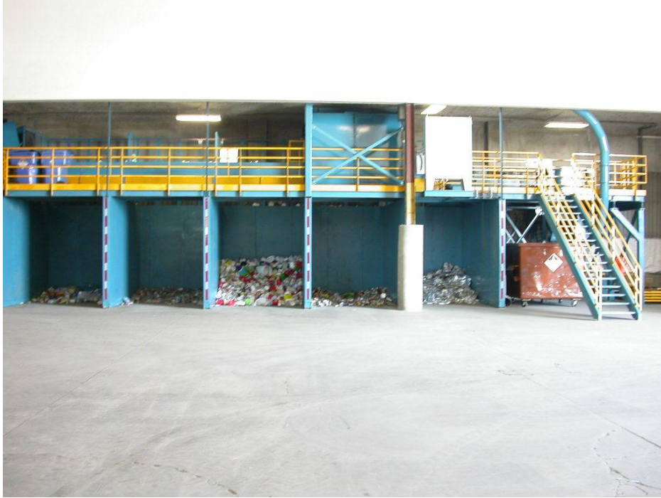
Photo of the new container line that was installed at the Recycling Center at 112 Patton Street, North Bay, Ontario.
