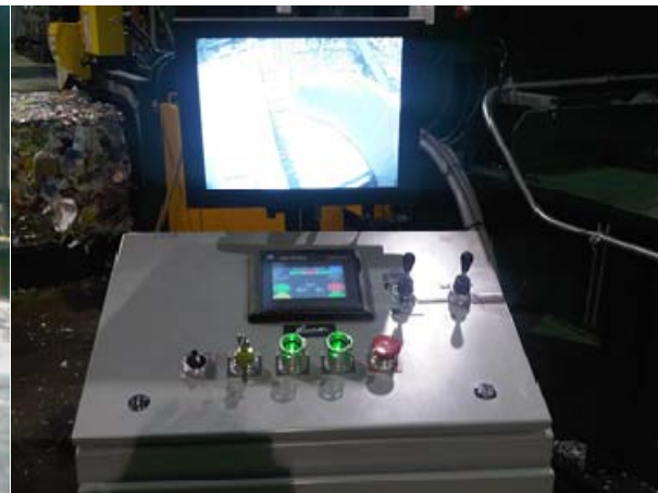
Photo 4- Programmable Control Panel
